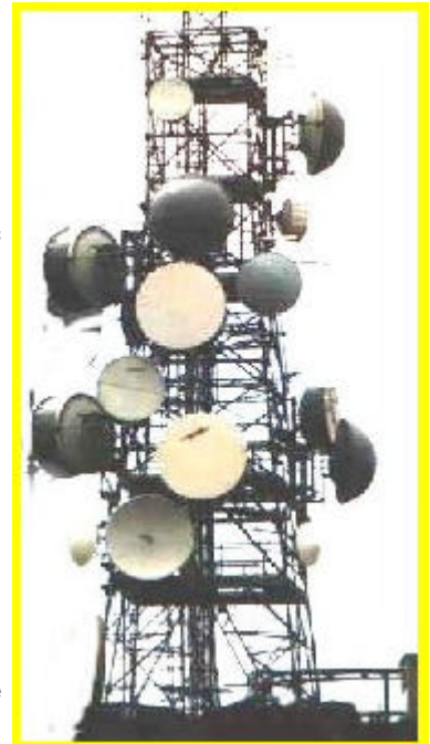
Inter-city microwave radio relay tower "spills" its signals into space (below)
